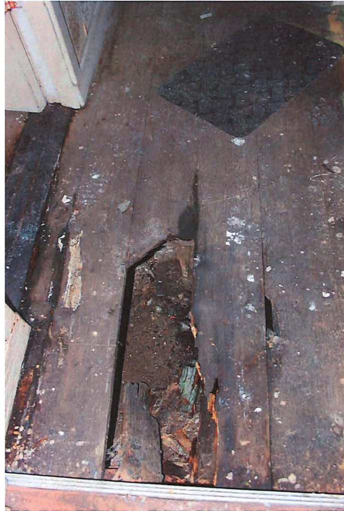
Fig. 29— Room 2-02, section of timber floorboards is missing.
