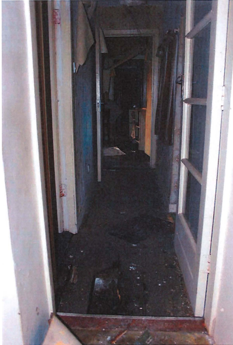
Fig. 26– Room 2-02, looking north. Section of timber floorboards is missing, wall paper finish is detached from the walls due to moisture.
