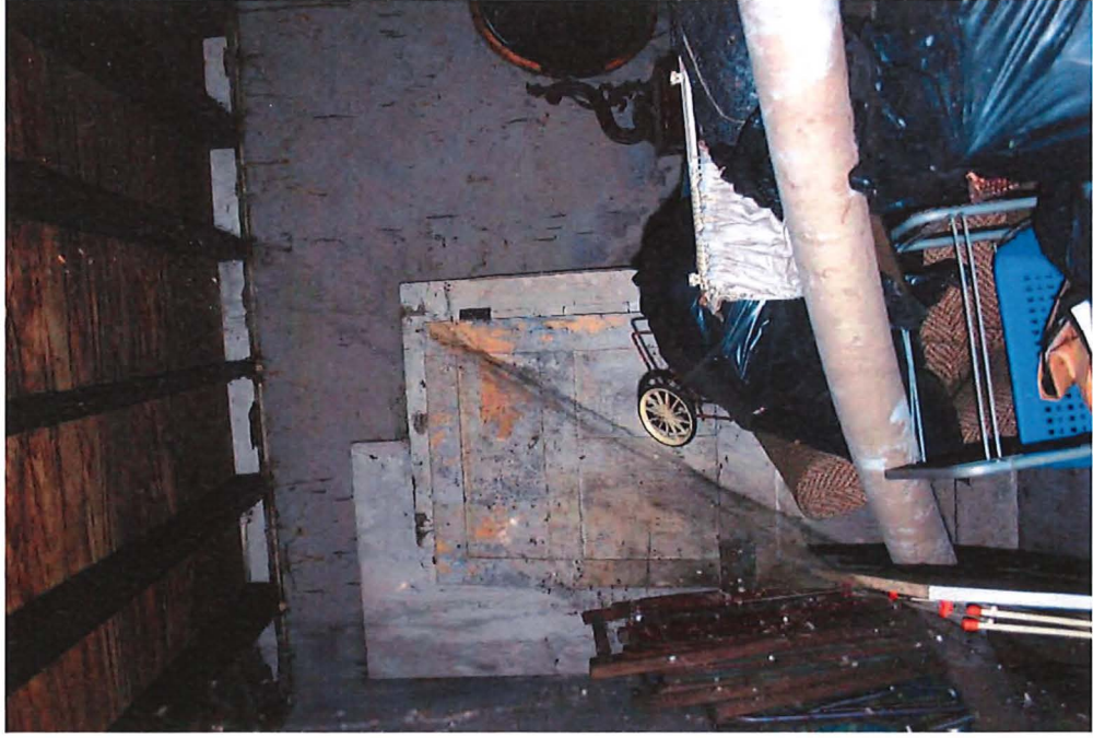
Fig. 56 – Room 3-05, looking west, non-original doors are dismantled.
