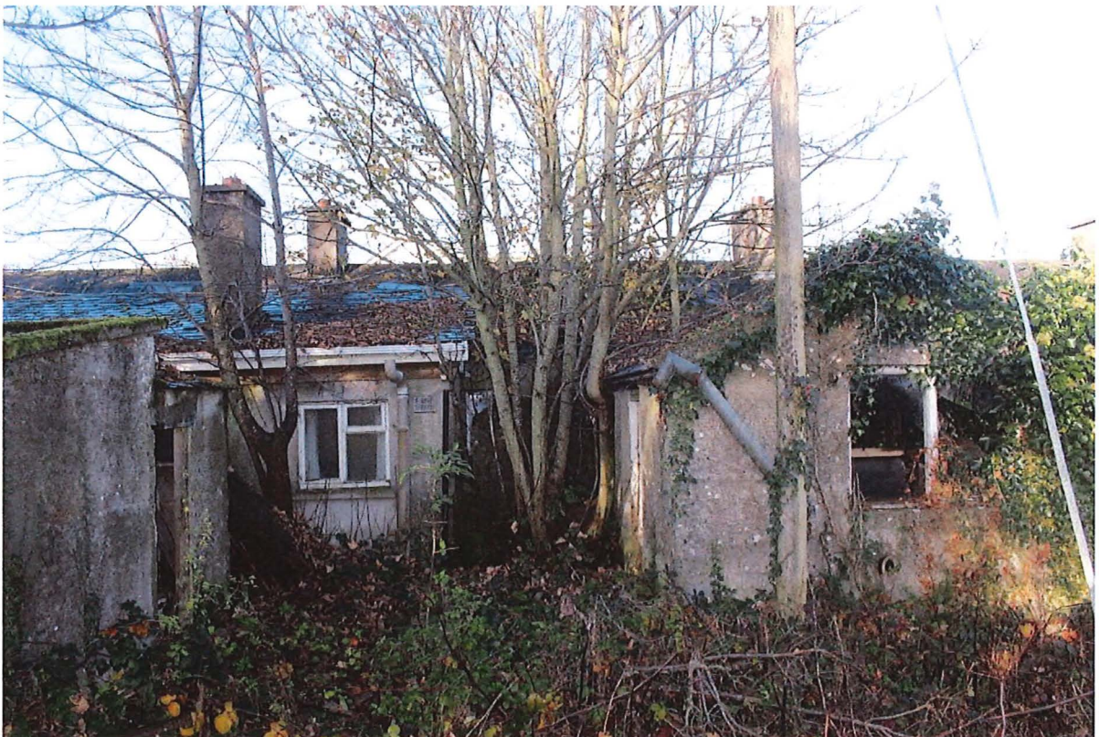
Figure 18: Rear of the cottages with modern extension at the back.
