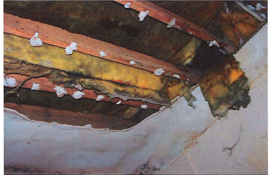
Fig. 16 – Room 1-04, the ceiling plasterboard finish collapsed. The wool insulation is exposed.
