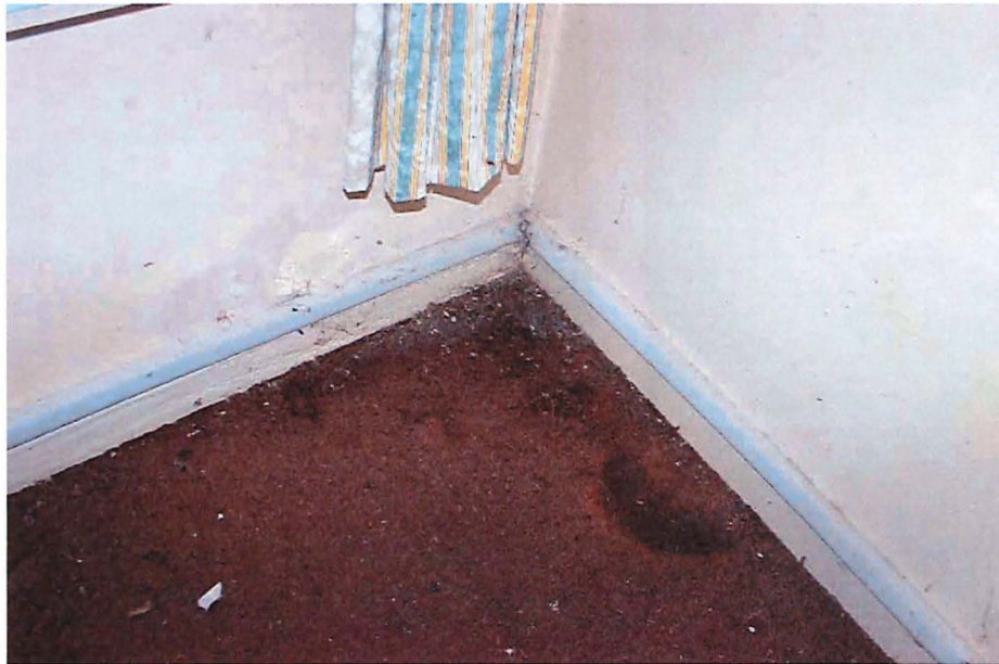
Fig. 51– Room 3-04, looking northwest. The carpet finish floor shows signs of moisture
