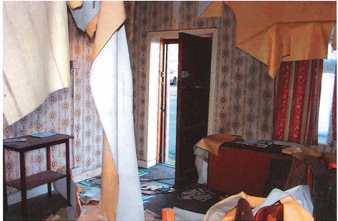
Fig. 37– Room 2-06, looking west, wall paper is detached from walls due to moisture.
