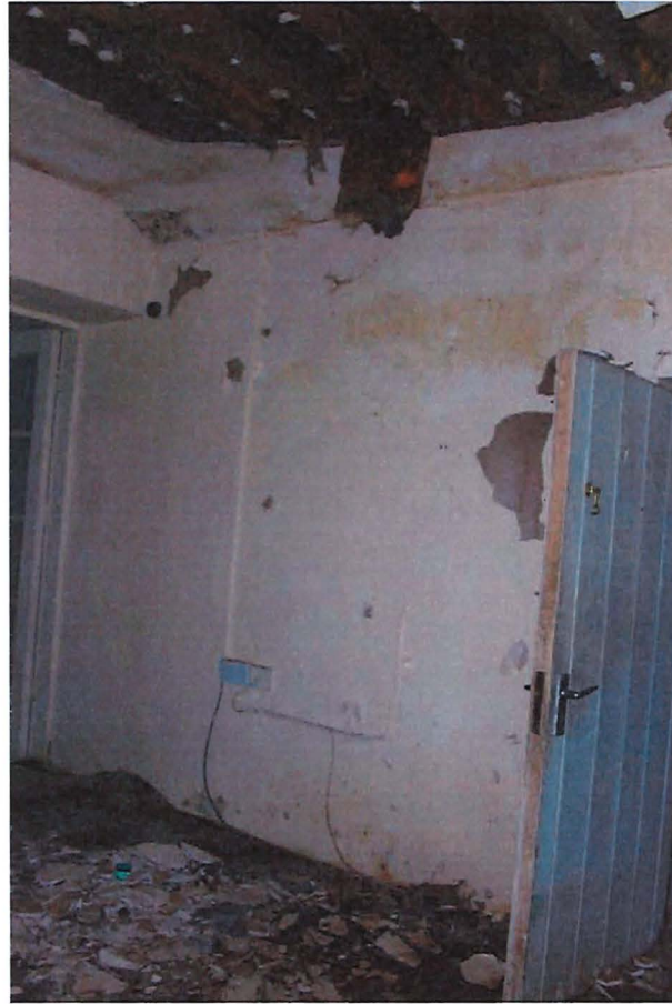
Fig. 10 – Room 1-04, looking northeast. The ceiling plasterboard finish collapsed. The wool insulation is exposed.
