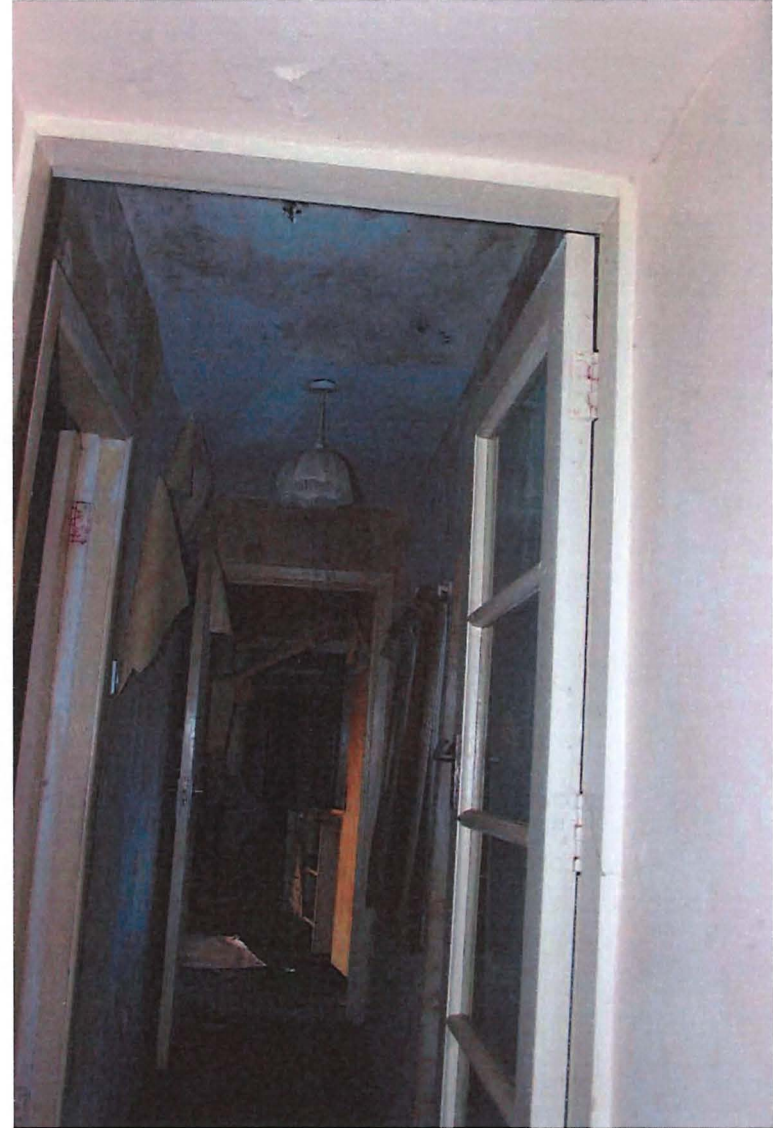
Fig. 27– Room 2-02, looking north. Plasterboard ceiling finish shows signs of moisture.
