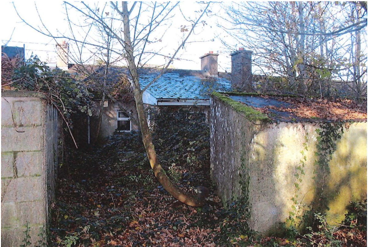
Figure 17: Rear of the cottages with mod-20 th century extension at the back.
