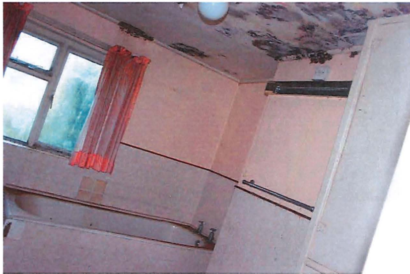
Fig. 30– Room 2-03, looking east, mid-20 th century extension bathroom, black stains on the plasterboard ceiling due to moisture.
