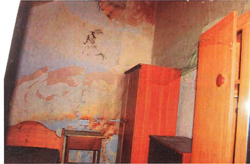
Fig. 5 – Room 1-02, looking south. Wall paper is detached from the wall and the plaster is crumbling (to the right) due to moisture.
